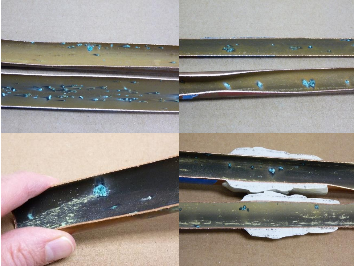
Figure 11: Images of Corrosion Pitting in Harvested Copper Pipes
