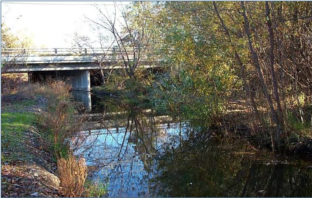
Example of a bridge over a perennial stream that maintains a natural bottom and accommodates wildlife passage.
