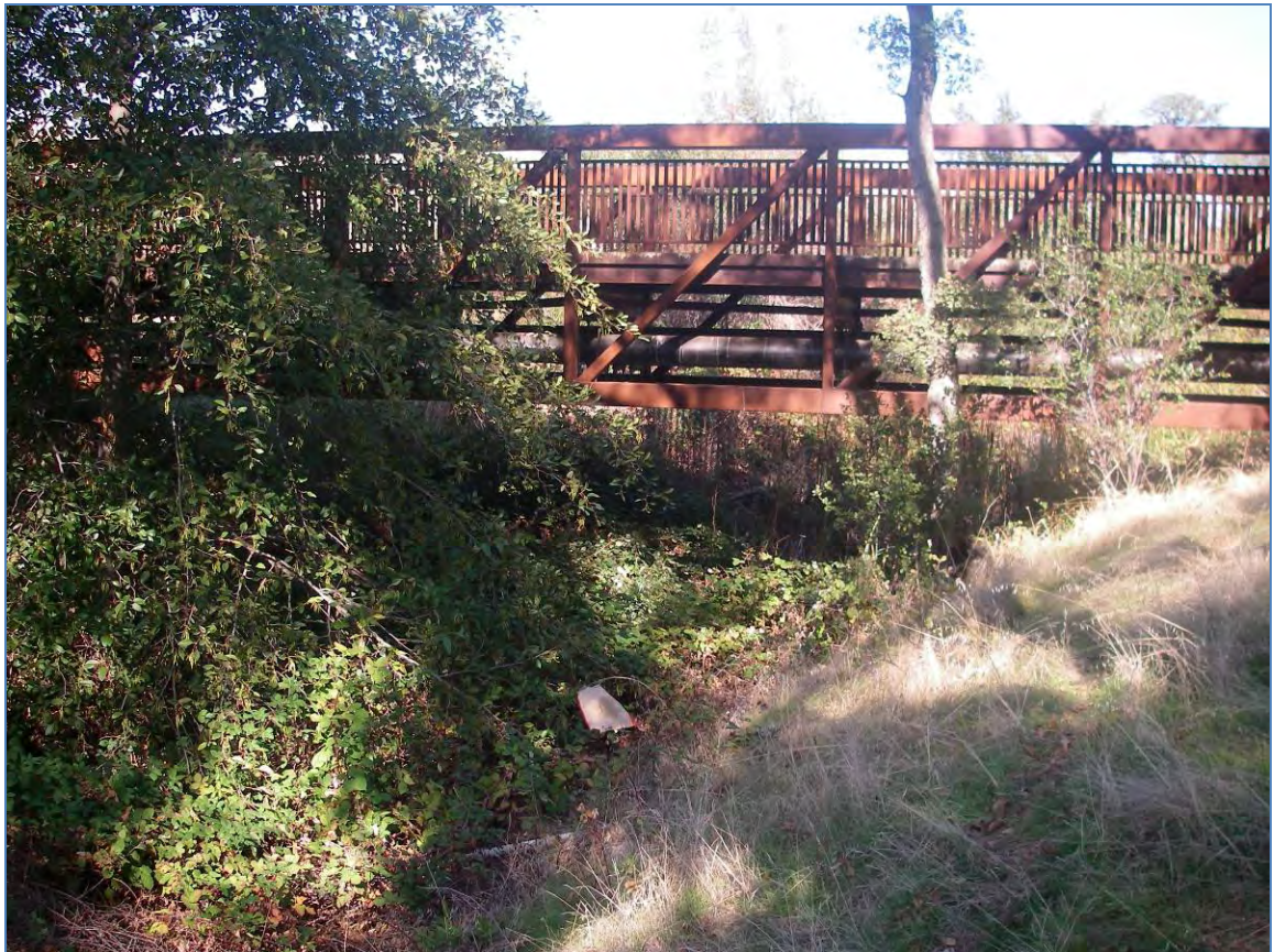
Clear span bridge with utilities attached shows the preferred method for utility crossings to minimize impacts to the natural resources.
