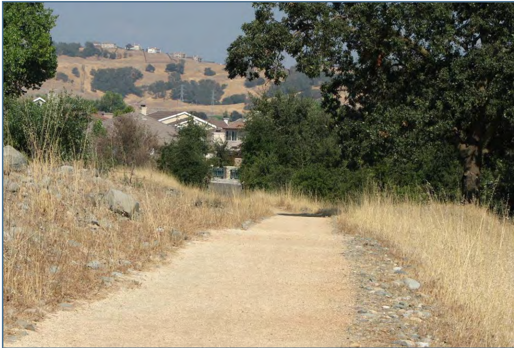
Outsloping the trail surface allows runoff to flow in sheets across the trail.
