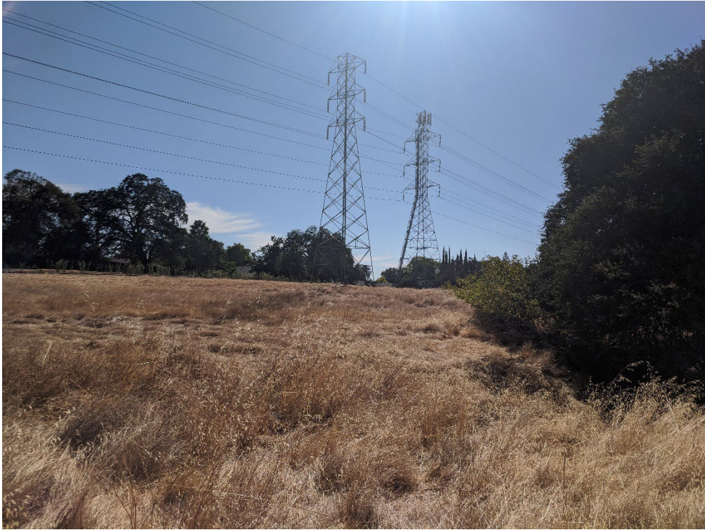
Photo 5: View of electrical towers along the southern boundary of the project site. Photo taken facing southwest.
