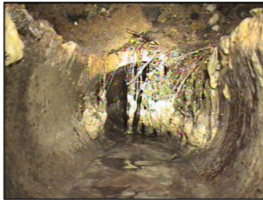
Grease Coated Pipe
